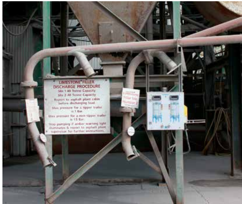
Delivery truck drivers can easily read the display panel while filling limestone dust into the two storage vessels.
