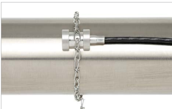
PT100 transducer fixed to pipe
